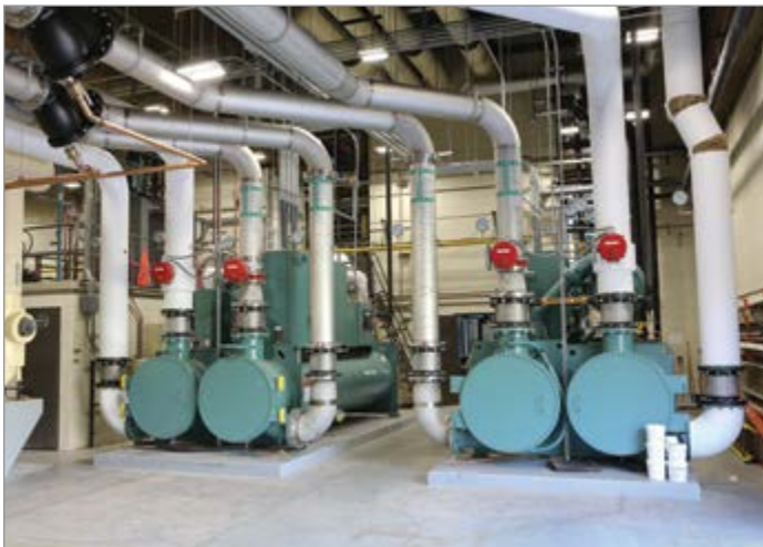
Magnetic bearing centrifugal chillers at the Hershey Medical Center’s central chiller plant.
