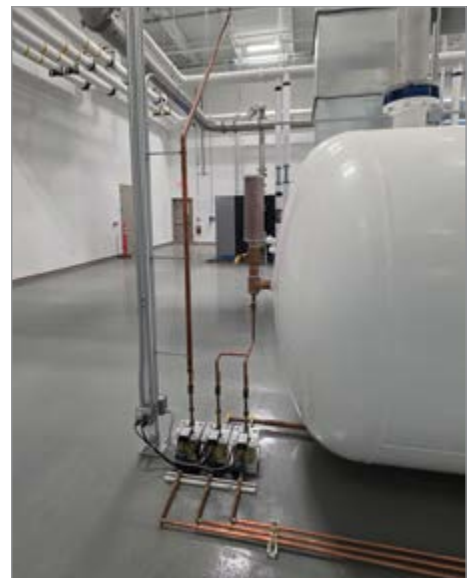
Add a condensate drain before the wet-side header, and two condensate drains to any wet tank.
