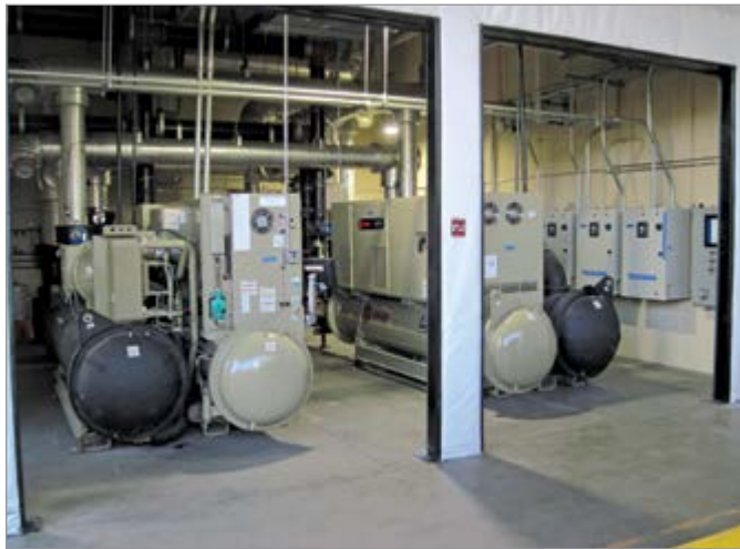
Variable frequency drives are now common in utility systems.
