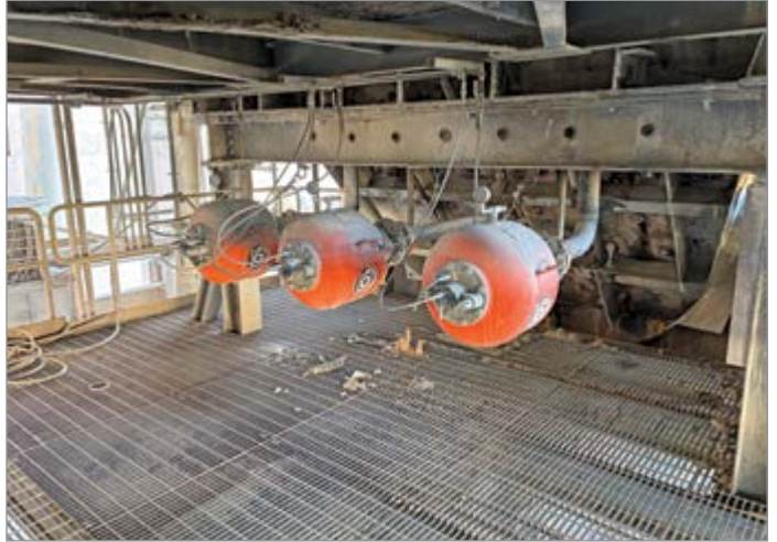
This older kiln blow-off system, which used 100 scfm of compressed air, was replaced with a new kiln blow-off system that included air cannons using 30 scfm of compressed air.
