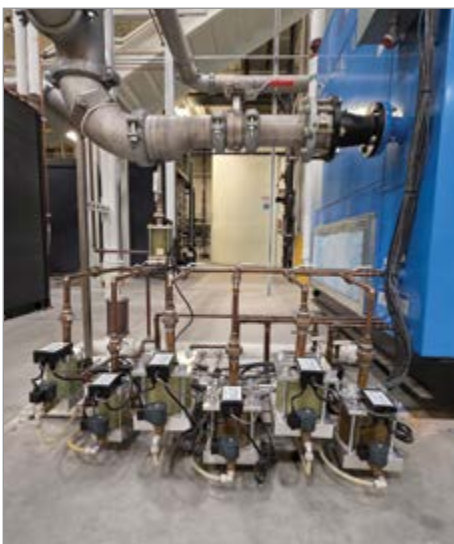
This two-tier condensate drain system offers full redundancy.
