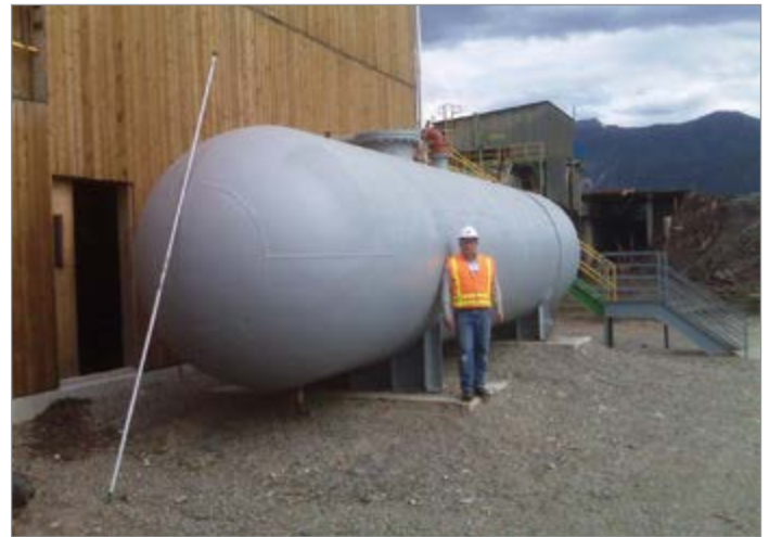
Dusty Smith, P.E., Director of Engineering, Pneu-Logic, stands in front of an air receiver installed to help deliver large volumes of compressed air instantly to meet sudden process demands.
