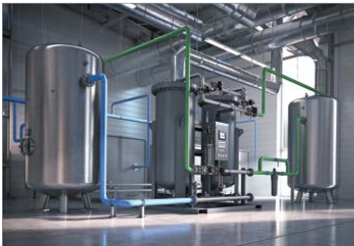
Inside a modern air compressor room at Atlas Copco, where advanced engineering meets efficiency.
