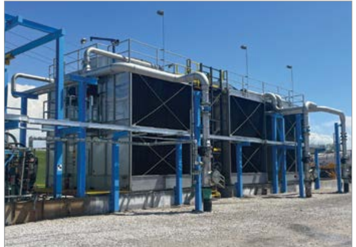
Midwest Machinery engineered a three-cell, double-stack, dual air inlet, crossflow, factory-assembled cooling tower on the old cooling tower’s foundation.
